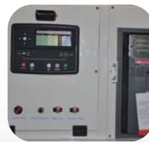
Control Panel & MCB
